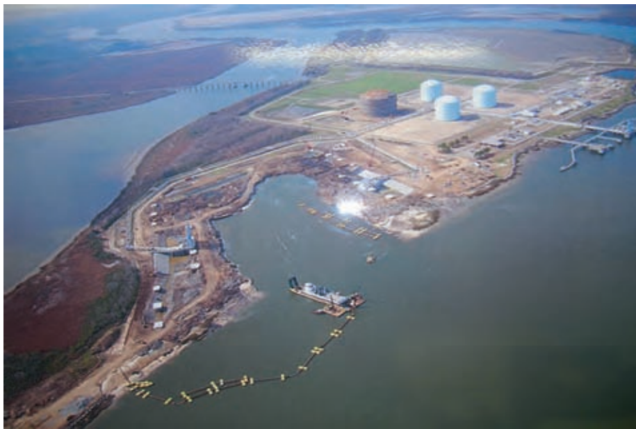
Southern Natural Gas Company's LNG facility expansion project at Elba Island, GA.
