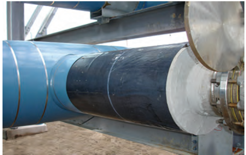
Vapor retarder mastic coating over ISO-C1 at termination. Aluminum jacket adds mechanical protection to the insulation system.
