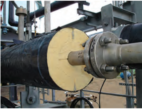
Staggered, double-layer ISO-C1 polyiso, terminating at flange. Joint sealant on outer longitudinal seam; vapor retarder sheet.
