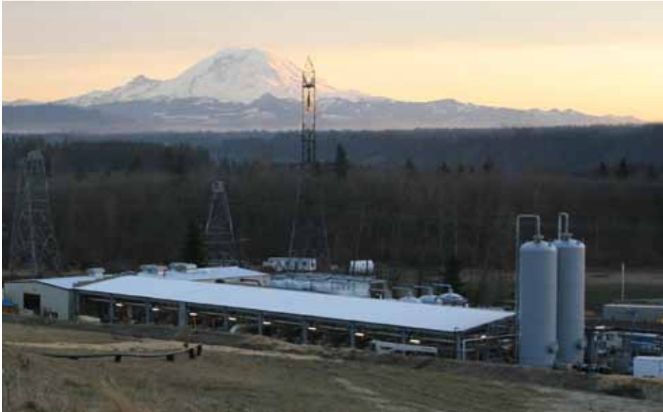
The Low-Profile Cedar Hills Landfill Gas Facility near Seattle, with Mt. Rainier in the Background
